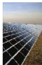
Large Thin Film power plant.
