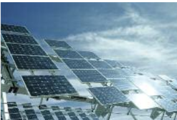
PV power plant in Darro, Spain.
