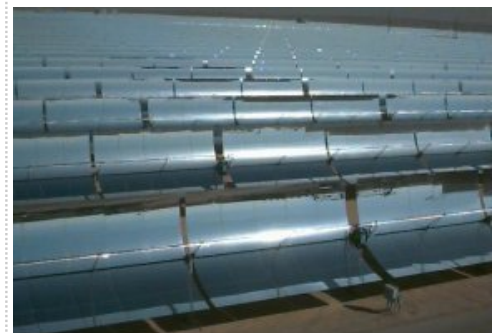
Parabolic trough power plant
