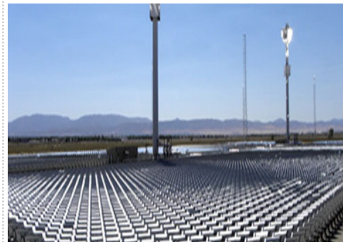
Solar power tower
