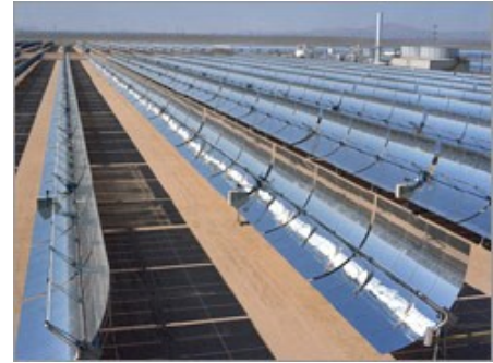
Array of parabolic troughs.
