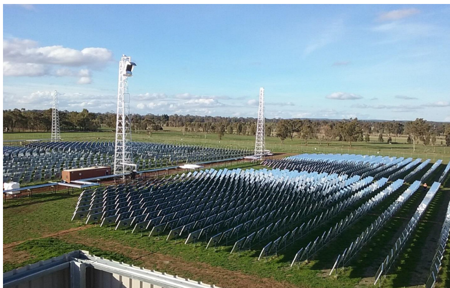
Fig. 16. Construction of the Vast Solar 6 MW e sodium power plant at Jemalong Solar Station, Australia. Source: C.K. Ho, Sandia National Laboratories.
