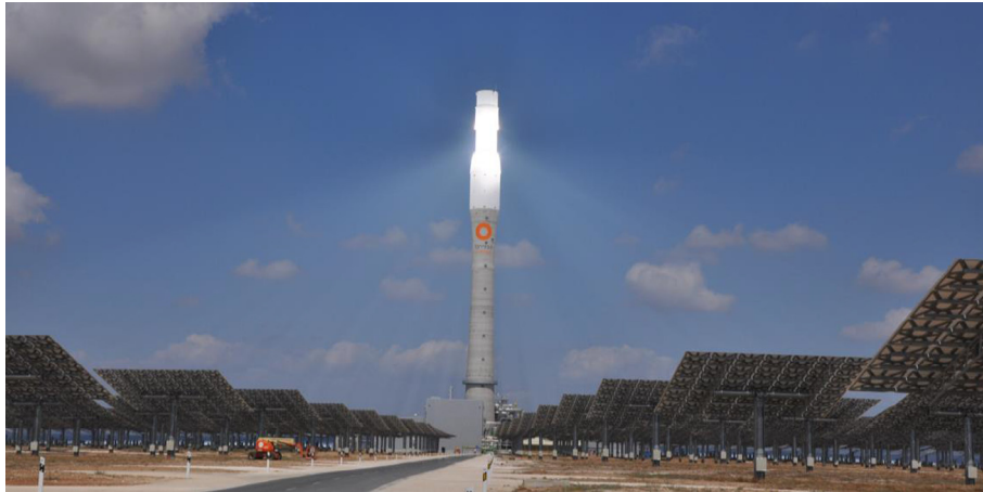
Fig. 6. Gemasolar molten-salt power tower near Sevilla, Spain. Source: C.K. Ho, Sandia National Laboratories.
