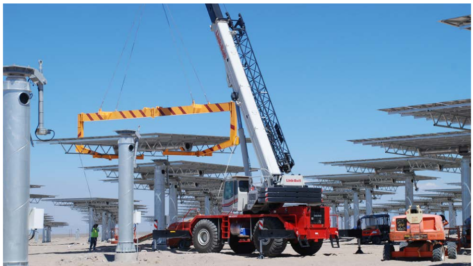
During construction of Crescent Dunes , 600 jobs were created. Photo Credit: SolarReserve, LLC
