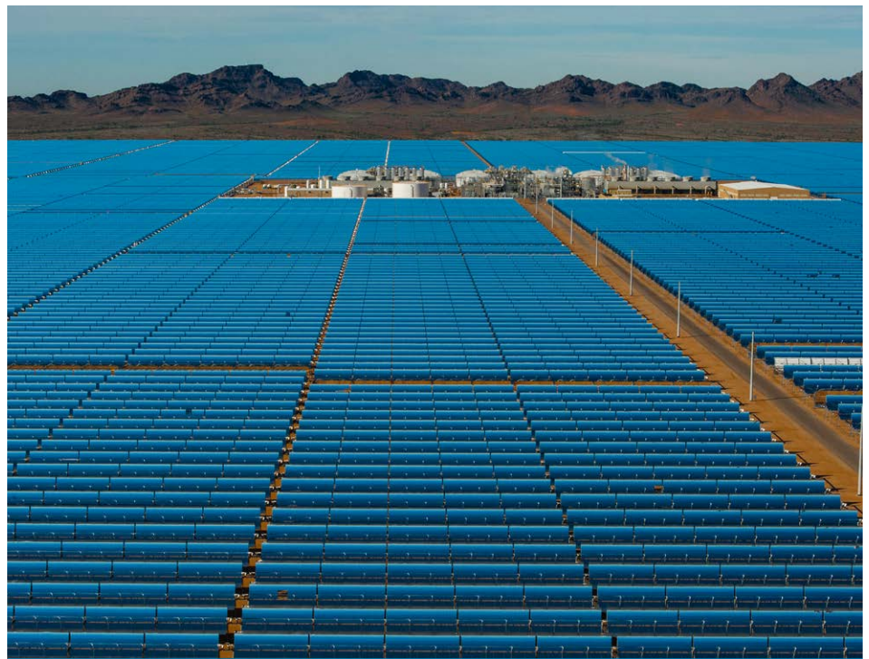
The Solana parabolic trough and thermal storage plant spans 1,920 acres near Gila Bend, Arizona.
