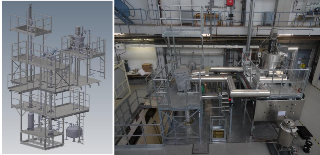
FIG. 5. The COMPLIT facility: principal layout and a picture of the installed facility
