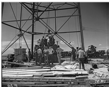
The explosives of "the gadget" were raised to the top of the tower for the final assembly.
