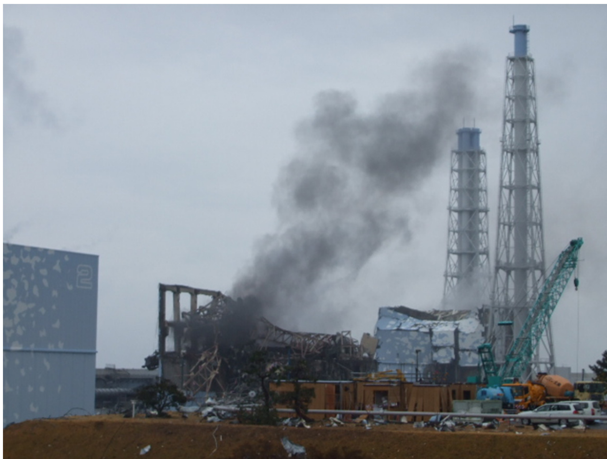
FIGURE 3.9 March 21, 2011, photo of damaged Unit 3 (middle) and Unit 4 (right) reactor buildings. Unit 2 is shown on the left margin of the photo. SOURCE: Courtesy of TEPCO ( http://photo.tepco.co.jp/en/date/2011/201103-e/110321-01e.html )
