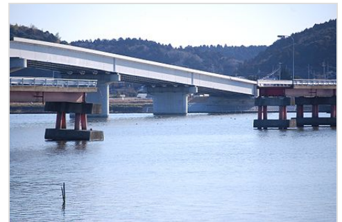
A highway bridge damaged and severed
