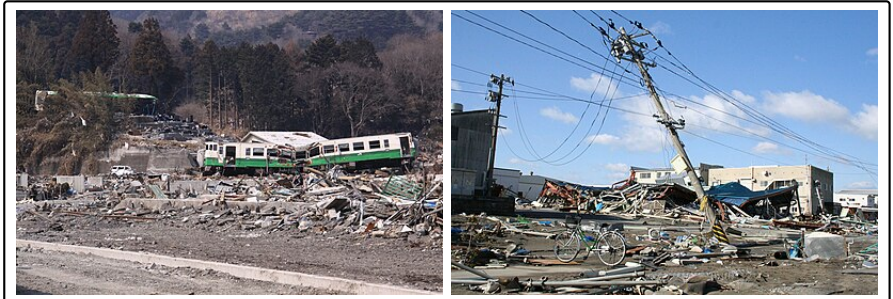
A KiHa 40 series train washed away uphill from Onagawa Station (left) and a damaged utility pole in Ishinomaki
