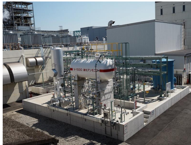
Ammonia supply unit
