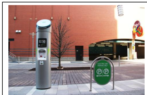
Figure 6. Example of a 240-Volt Commercial Charging Station Installed by IPL
