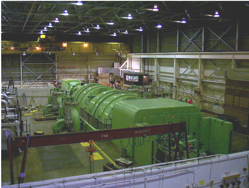
Monticello nuclear generating plant turbine deck [29].
